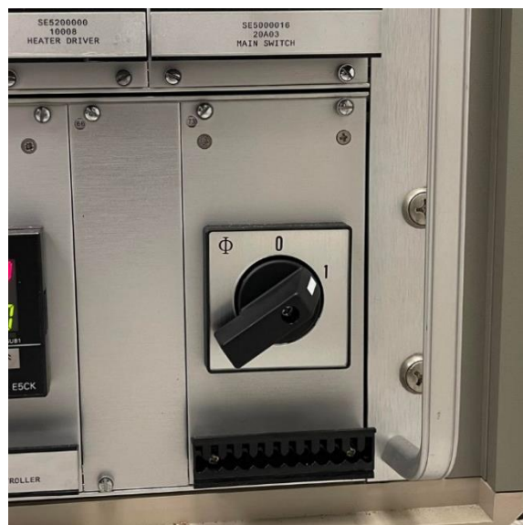
Figure 2. Heater Power Switch for EVG 501
