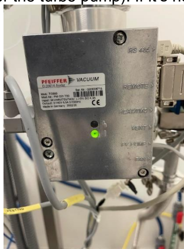
Figure 27. Turbo pump power supply in working condition.
